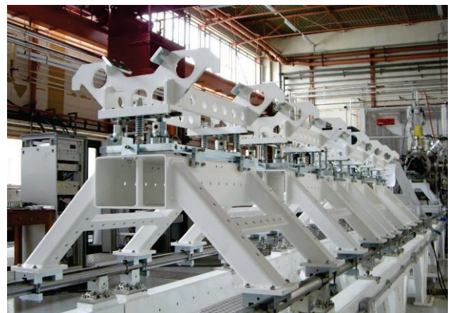
Figure 5: Complete RFQ support system installed at RAL
